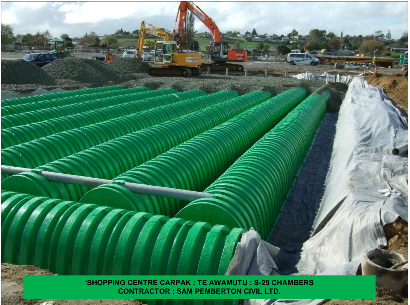
'THE BASE' SHOPPING CENTRE CARPAK : TE-RAPA HAMILTON : 1,700 S-29 CHAMBERS CONTRACTOR : SAM PEMBERTON CIVIL LTD.
