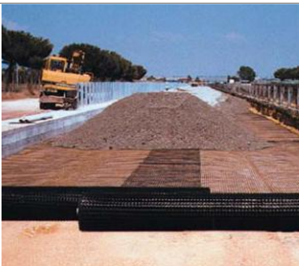
Road : Low Bearing Capacity SubGrade Reinf.
