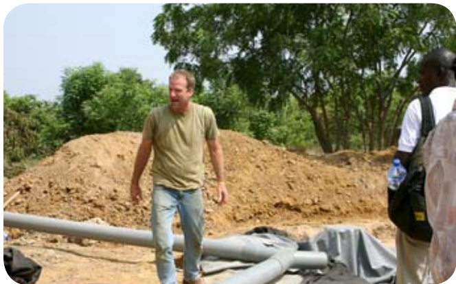
Underground pipe is installed to carry water from the downspout to the rainwater storage basin.
