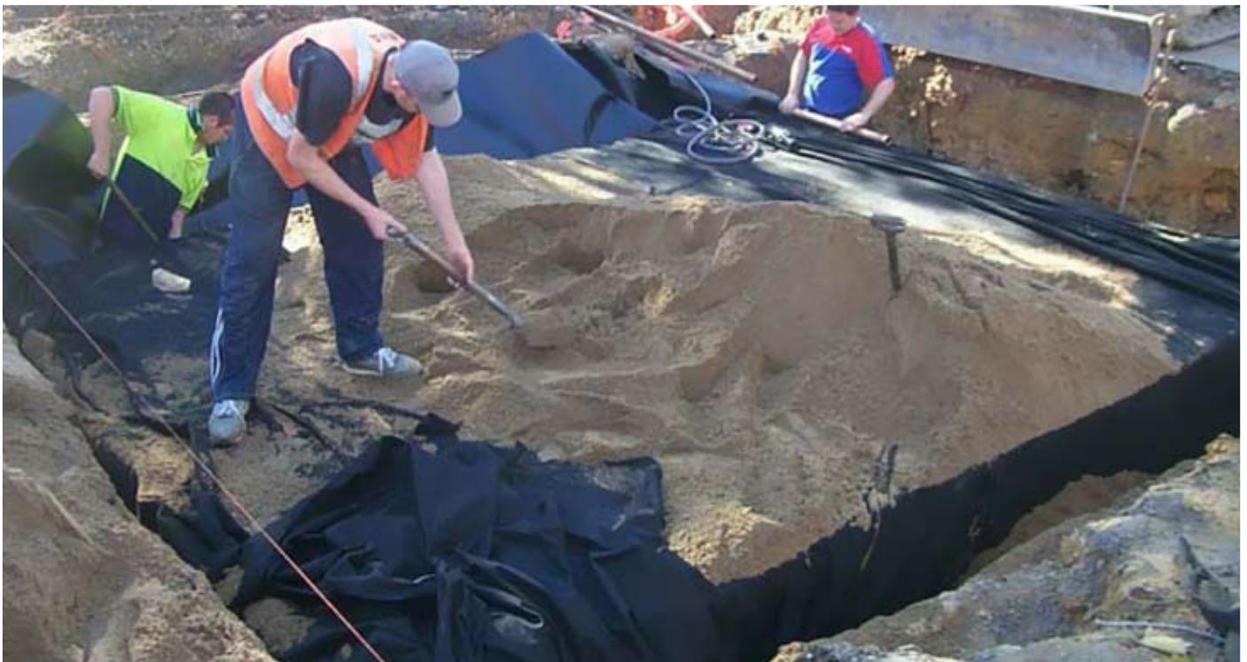
Following installation of tank and liners, sand was used for fill. Note the plumbing for drawing off water from the tank.
