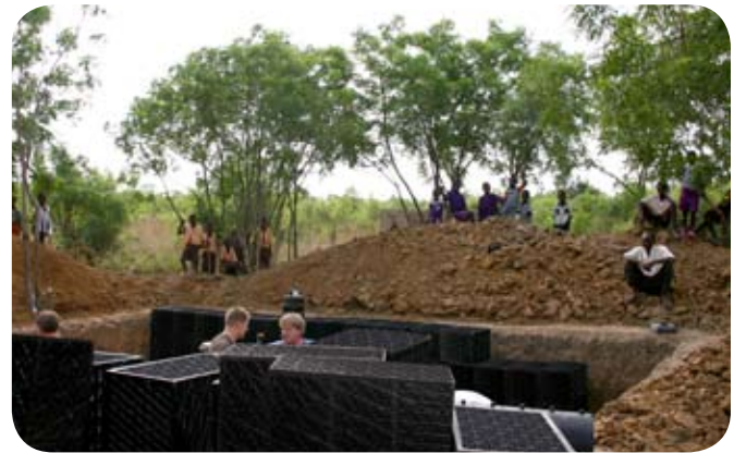
240 modular tank units are set into the basin creating an 8,000 gallon reservoir.
