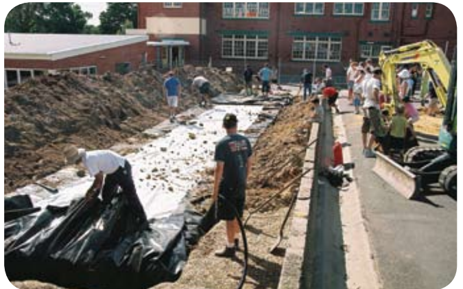
Finally pulling up the impermeable liner on all sides and taping it on top.
