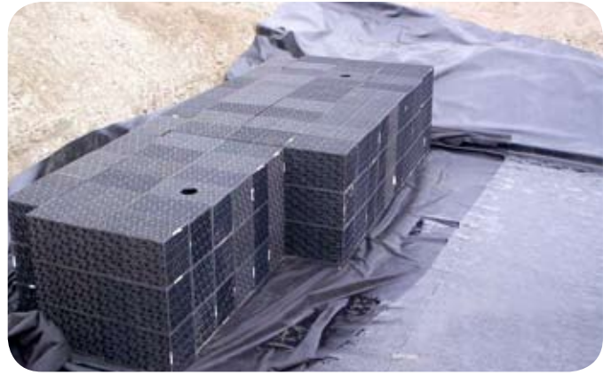
Installing the Atlantis® D-Raintank® (Matrix®) modules on top of the impermeable liner layer and the geotextile layer.
