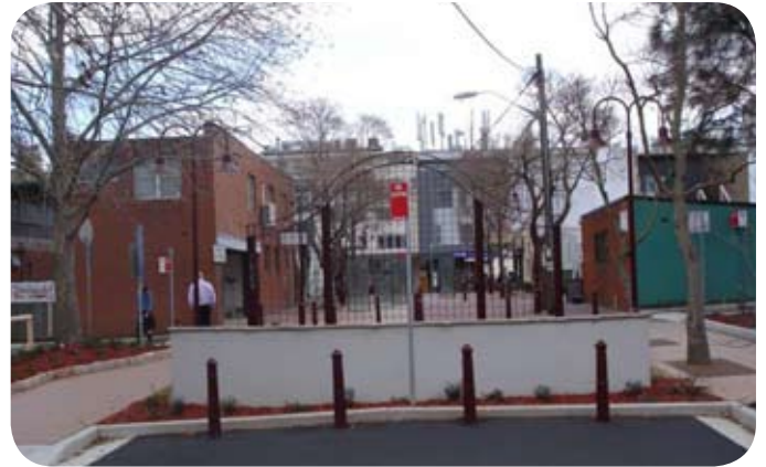
Looking west after installation. The electrical and pump stations are at far right.
