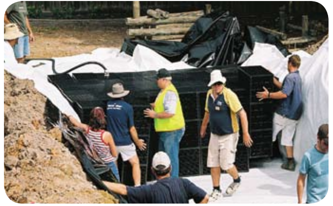
Installation of Geotextile lining and Tank Modules in the impermeable liner excavated area.
