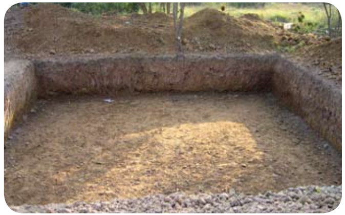
The 22' x 24' basin has a depth of 4 feet. 240 modular tank units will fill this hole.
