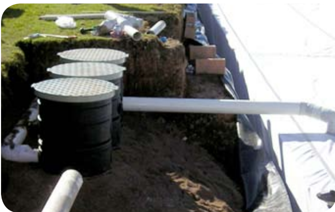
connecting inlets, outlets to filtration units.
