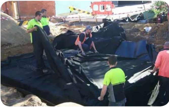
Following excavation the lining was placed, then the geofabric which wrapped entirely around the tank.
