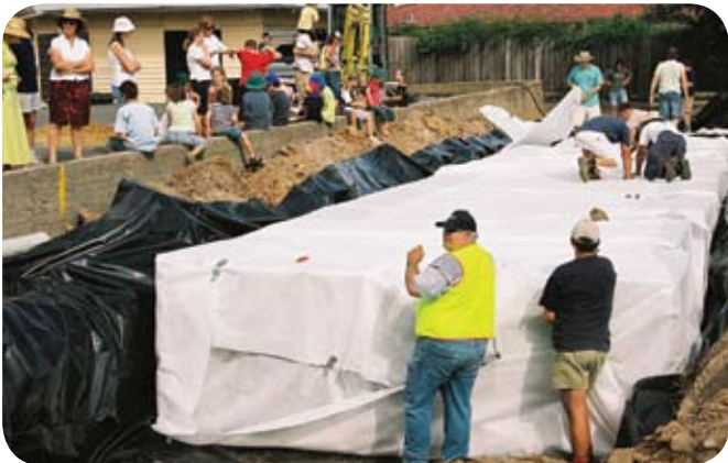
Completely wrapping the Atlantis® D-Raintank® (Matrix®) in Geotextile fabric and taping all the joints.
