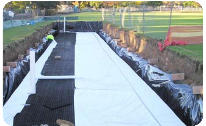
Pulling up the geotextile on all sides, taping it on top then installing and
